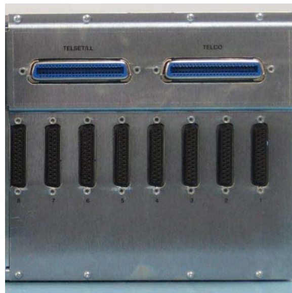
Figure 1-3. Example of Back Panel with 25-pin EIA DTE Connectors and Mass Termination Telco Connectors
